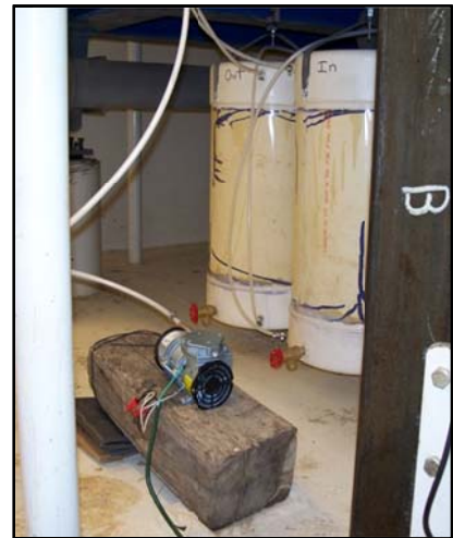
Figure 11. Vacuum pump and drainage tanks Photo by Dale Straw of DWR
