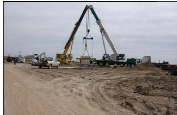
Figure 3. The inner tank plus soil being lifted off the ground prior to moving it to its permanent location
