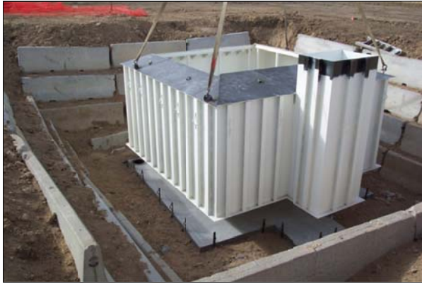
Figure 4. The outer tank being lowered into position. The concrete slabs were used to hold the soil in place. They were taken out before re-filling the empty space around the outer tank.
