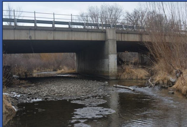
Bridge Opening Plugged With Sediment & Trees
